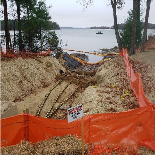
Fig 5: Trench and cable at Gundalow landing/east side of the Bay. Viewing west. (11-18-19).
