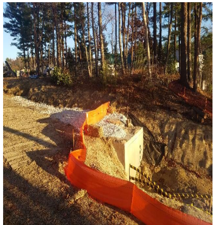
Fig 4: Stone placed on vault to raise surface elevation for New Rivers activities at Gundalow landing/east side of the Bay. Viewing south. (11-15-19).
