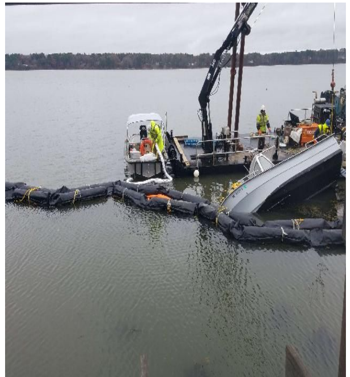
Fig 16: Deploying spill response absorbent boom around boat location to soak up any oil sheen on the water. Viewing east. (11-20-19).
