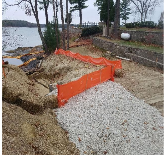
Fig 6: Stone added to raise ground elevation in order for New River to complete their work activities above the man hole at Gundalow landing/east side of the Bay. Viewing west. (11-18-19).
