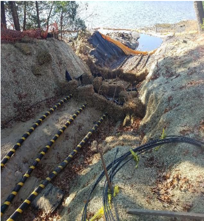
Fig 3: Sediment controls in trench at Gundalow landing/east side of the Bay. Viewing west. (11-15-19).
