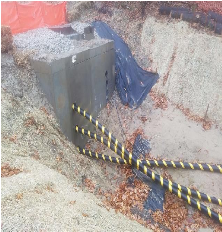
Fig 9: Cables assembled and secured in vault at Gundalow landing/east. Side of the Bay. Viewing southeast. (11-19-19).
