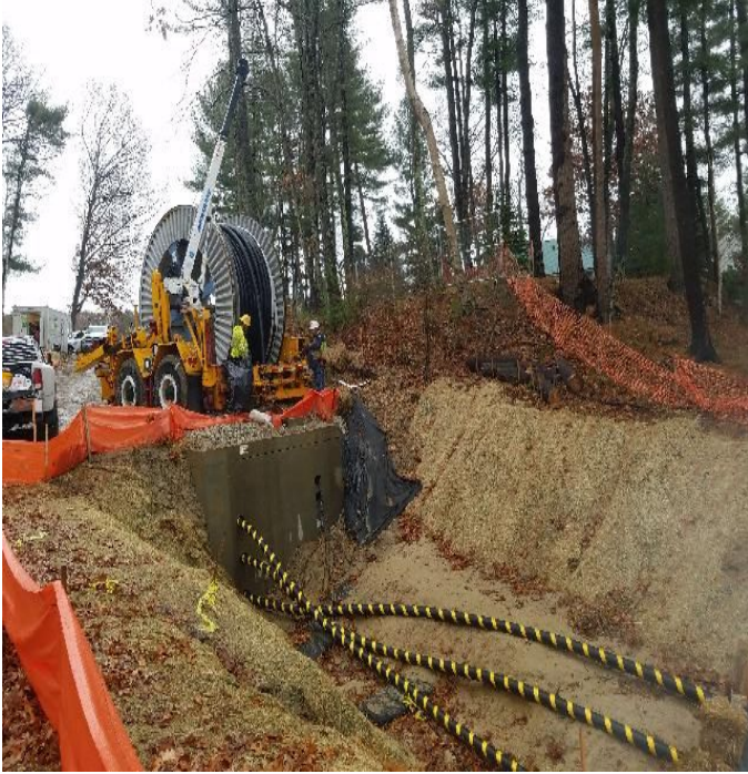
Fig 21: New River Electrical Co. pulling cable from vault at Gundalow Landing/east side of the Bay to riser Str. 100. Viewing east. (11-20-19).
