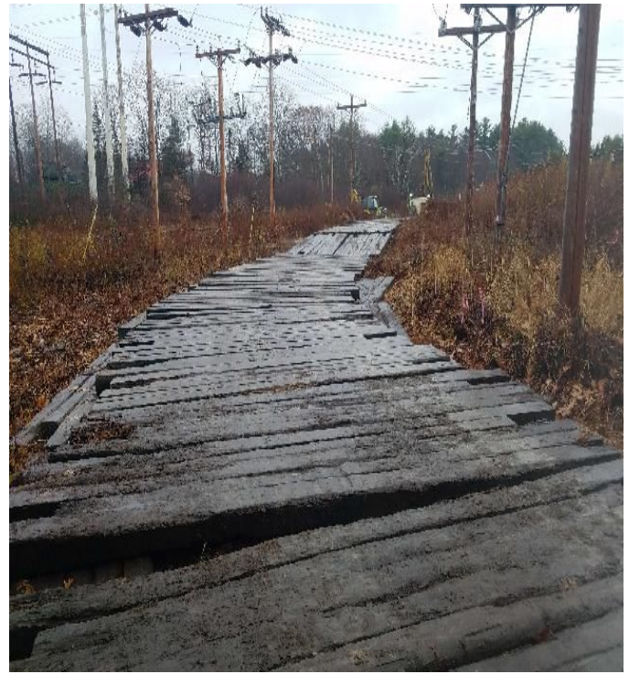
Fig 20: BMPs need to be installed along access in wetland MW2. Viewing south. (11-20-19).
